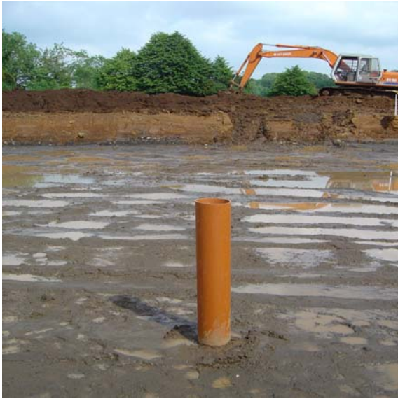
Figure 5 Pond 5 before flooding
